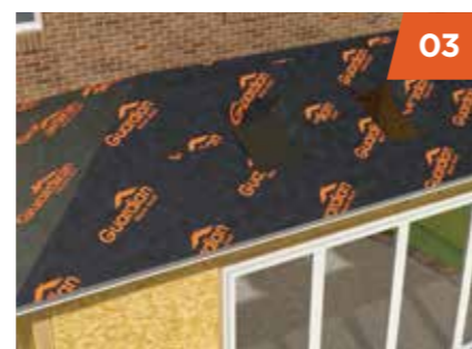
03 Breathable waterproof membrane is laid over the structural OSB 3 and secured in place.
