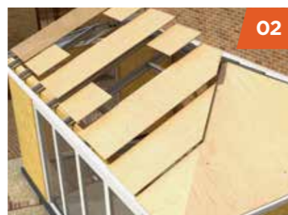
02 The aluminium roof structure is secured to the ring-beam and structural OSB 3 is fixed.
